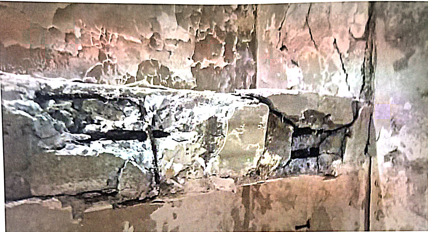
5. IN SHOP NOTICED BEAM HEIGHLY EXPOSED
