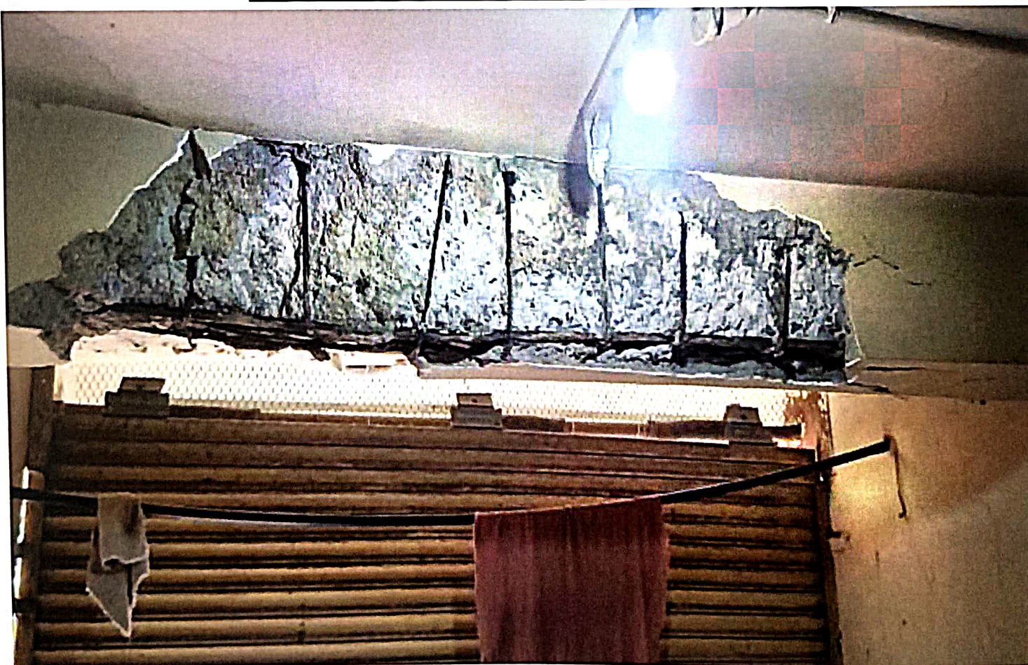
6. BEAM HEIGHLY EXPOSED HAS BEEN OBSERVED
