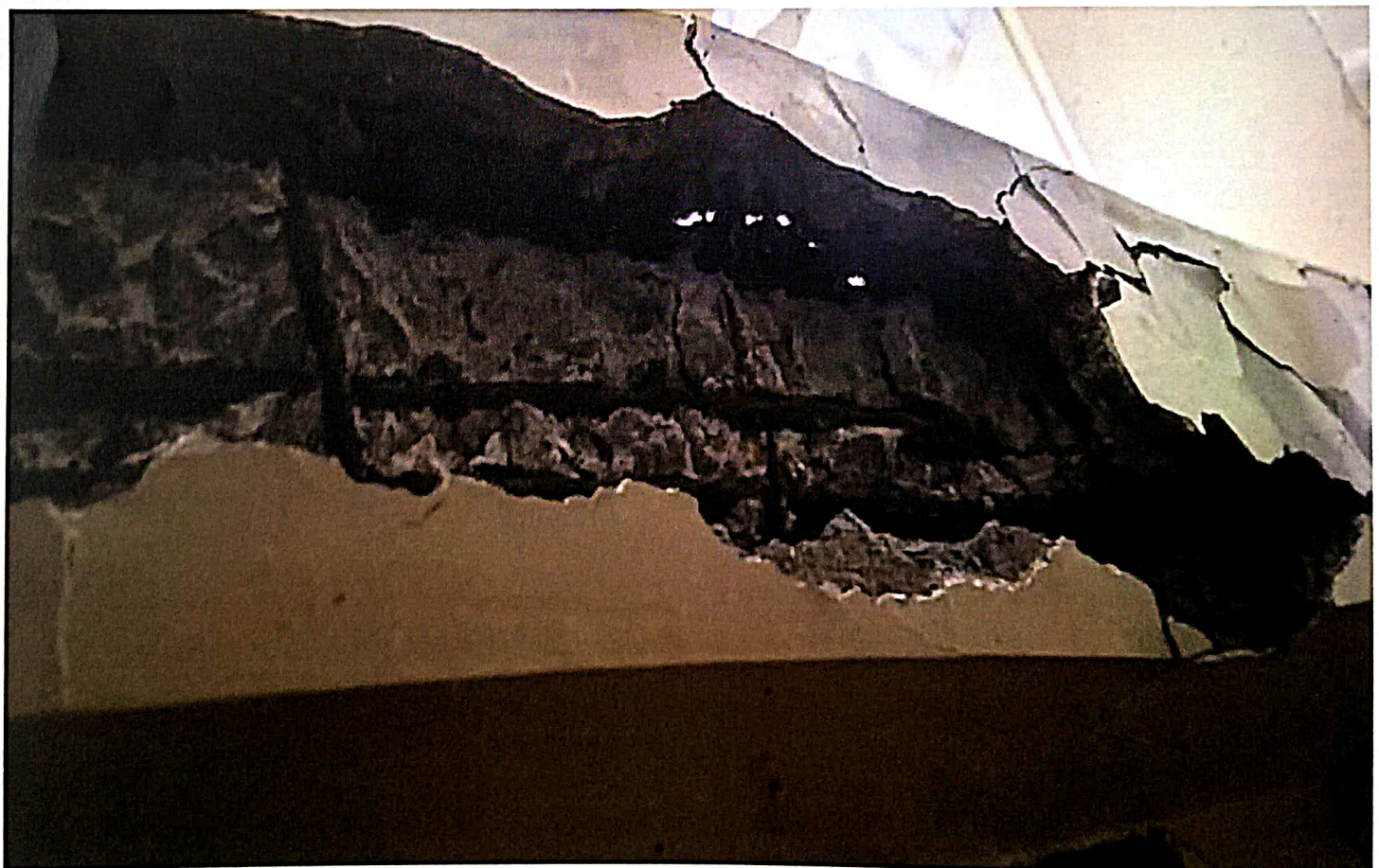
10. NOTICED BEAM HEIGHLY DAMAGED INSIDE THE GARAGE AREA
