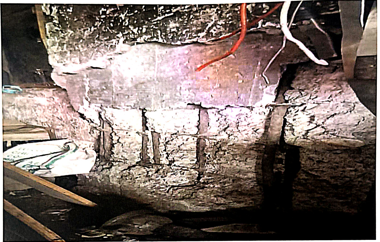
7. COLUMN HEIGHLY EXPOSED HAS BEEN OBSERVED .
