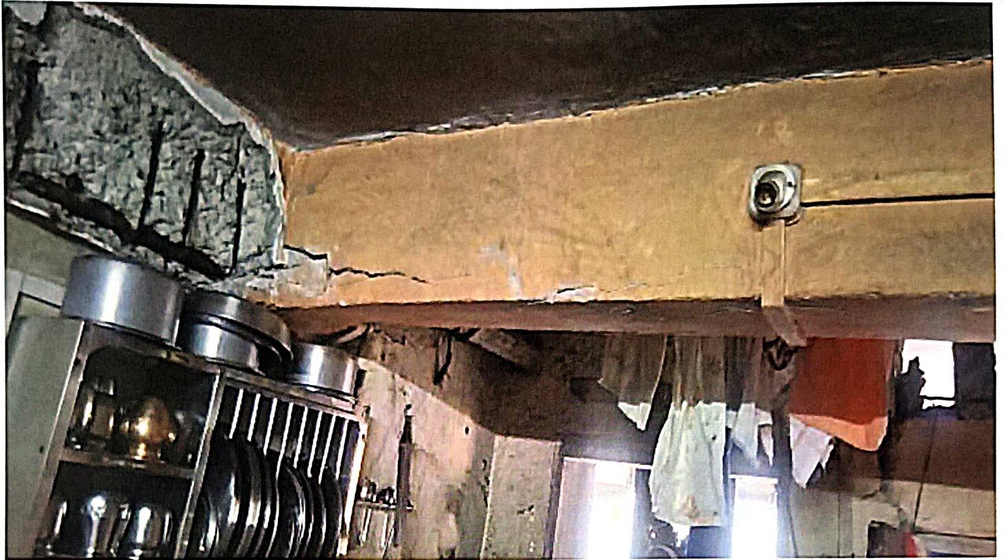
9. NOTICED BEAM HEIGHLY DAMAGED INSIDE THE GARAGE AREA
