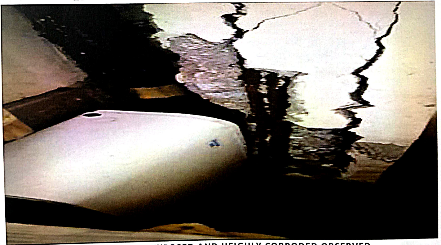
4. STEEL EXPOSED AND HEIGHLY CORRODED OBSERVED .
