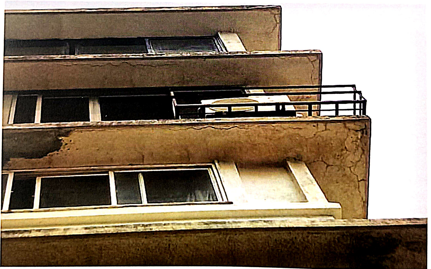
2. EXTENSIVE CRACK & FUNGUS OBSERVED ON THE EXTERNAL WALL PLASTER
