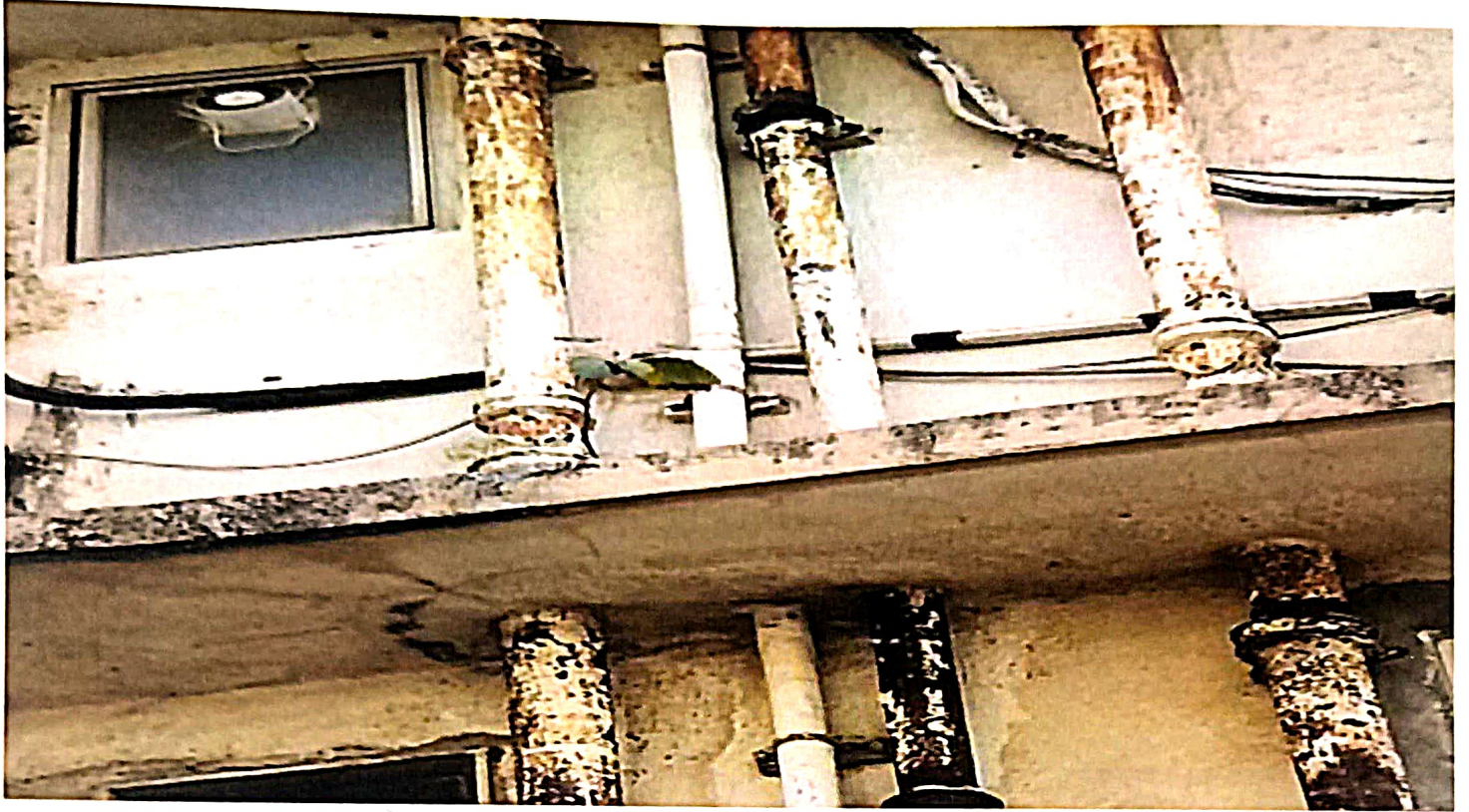
1. NOTICED VEGETATION GROWTH DEVELOPED AT EXTERNAL WALL AREA
