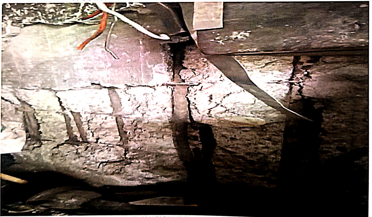
8. COLUMN HEIGHLY EXPOSED HAS BEEN OBSERVED
